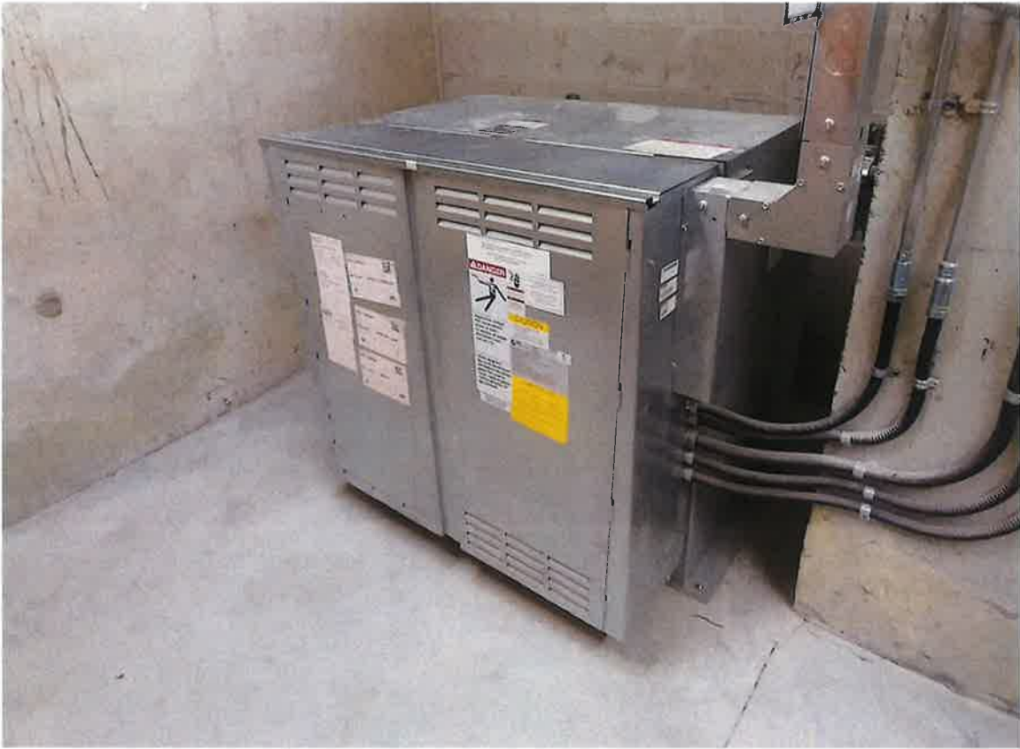
View of the elevator hydraulic fluid reservoir
