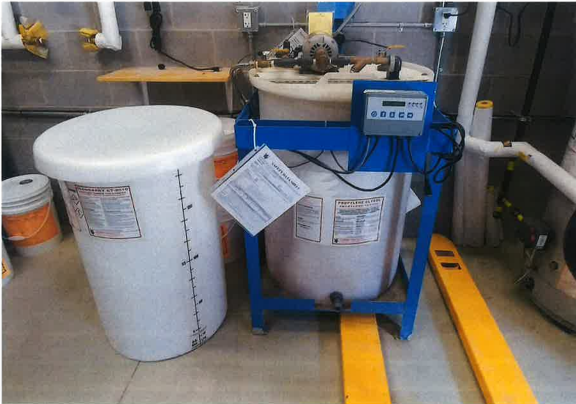
View of abandoned cooling tower water treatment system
