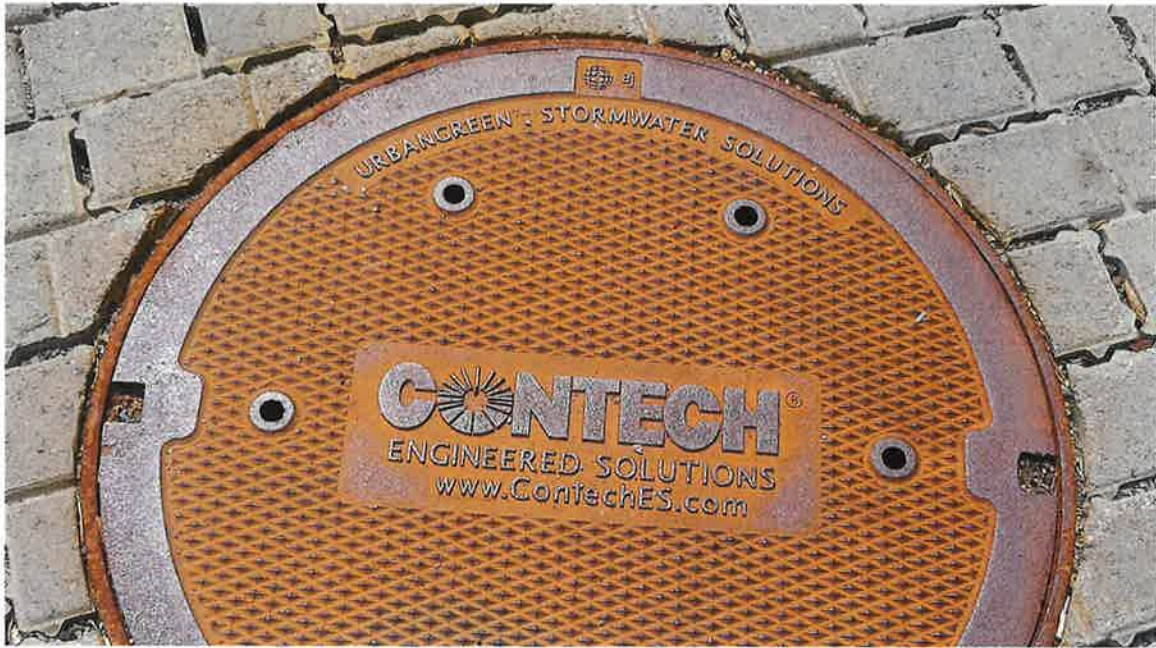
View of the cover of underground storm filter tank located in the parking lot
