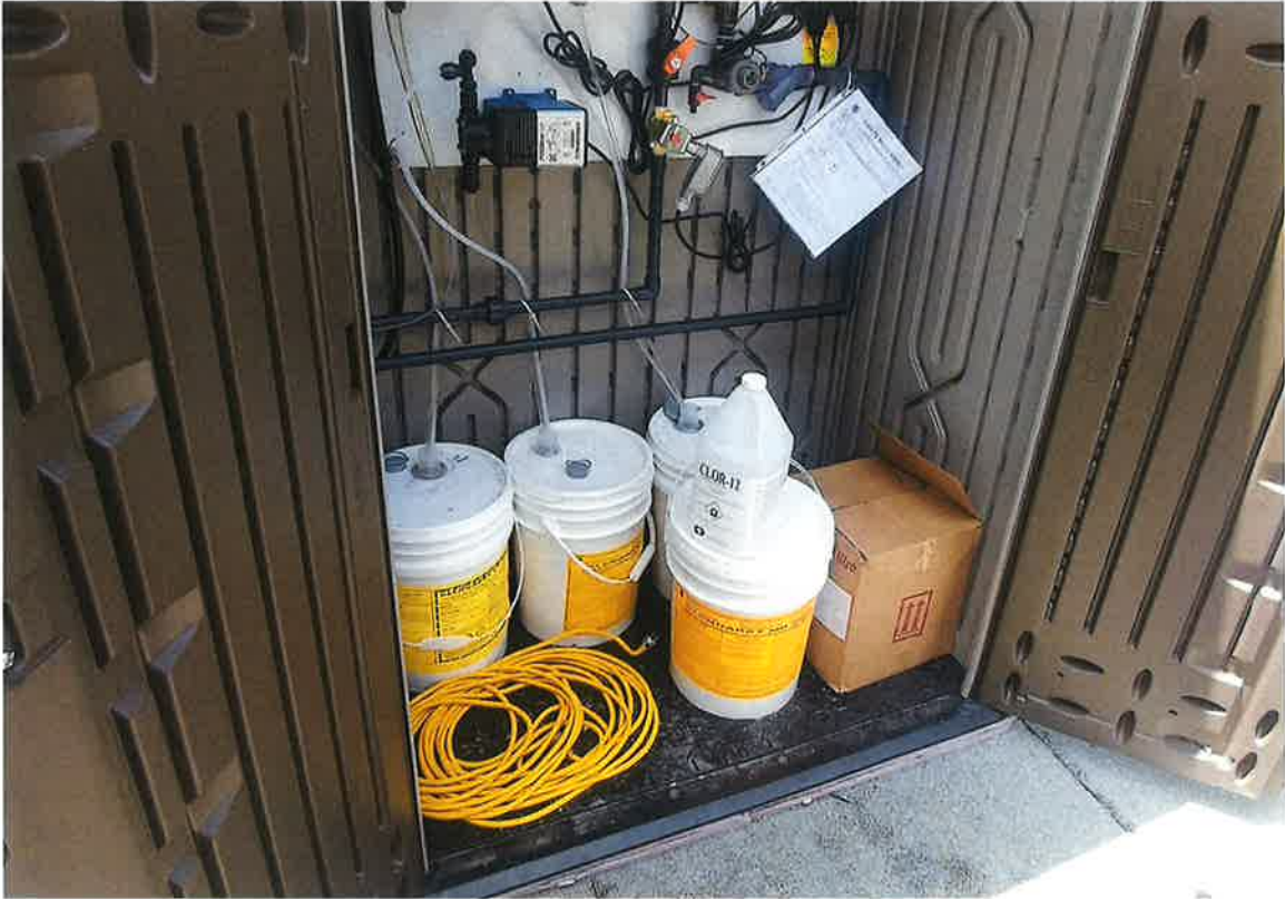
View of the roof mounted cooling tower water treatment system
