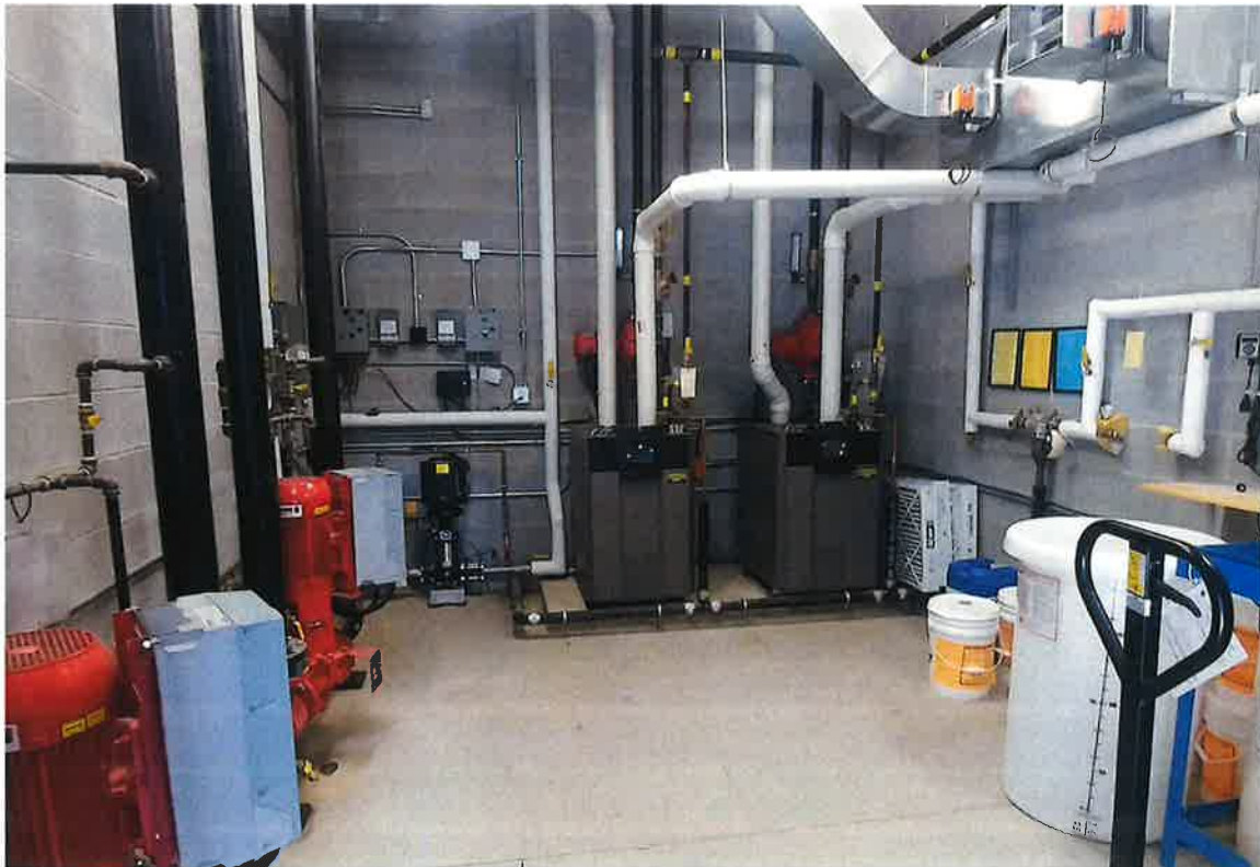
View of the mechanical room
